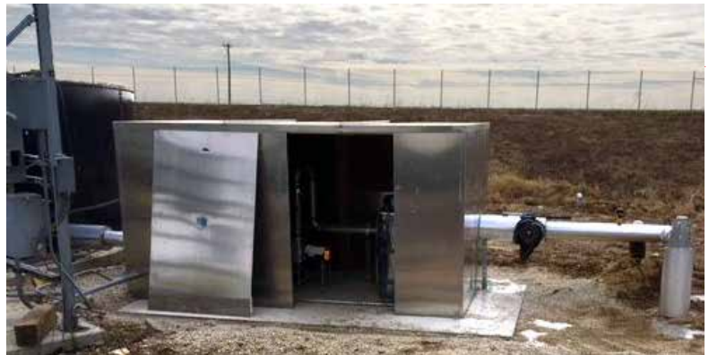
Figure 1: Leachate Lift Station
