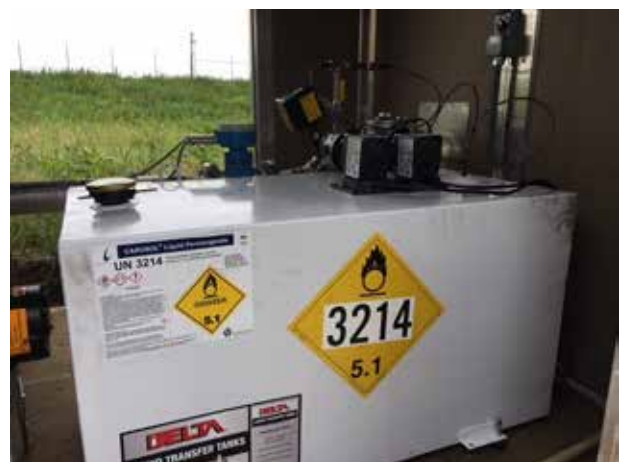
Figure 2: CARUSOL Tank and Metering Pumps
